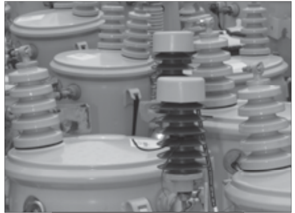
Thieves across the country are damaging electrical equipment like these transformers for the copper they contain. Some thieves are paying for the theft with their lives.
